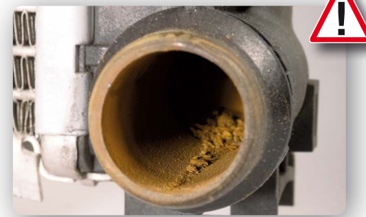
rust in the radiator
